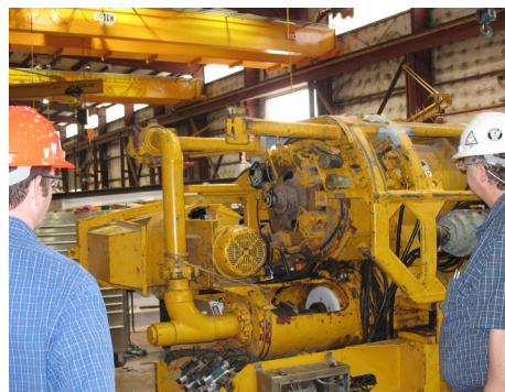
Encoder installed in gear box
